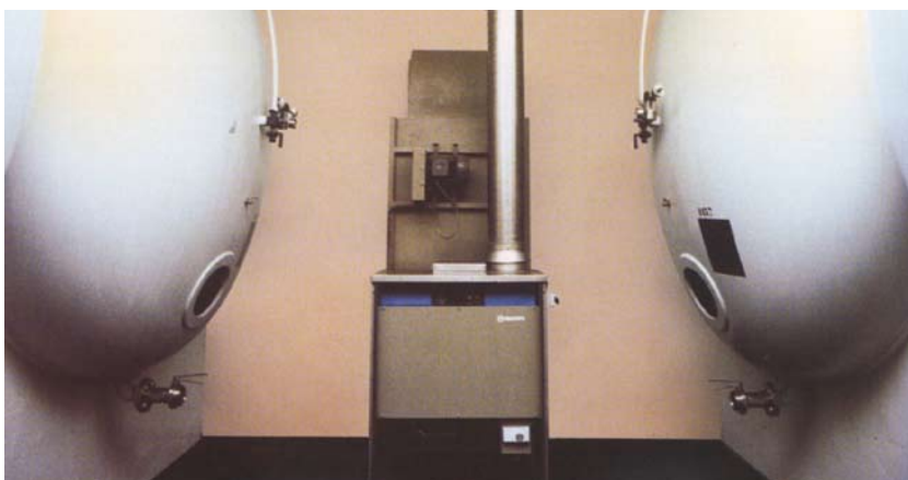
Controlling condensation on chilled tanks.
