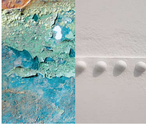
Old paint leaves the surface free for corrosion attacks. Applying new paint protects sensitive riveted joints for many years.
