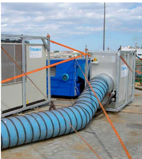
Dehumidifiers and chillers controlling climate in the cargo hold.
