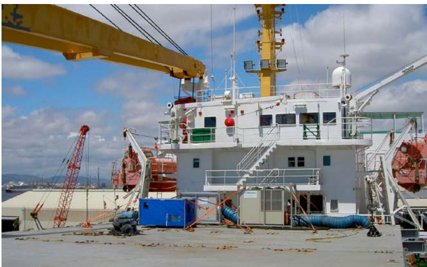
Temporary climate system for conditioning cargo hold.
