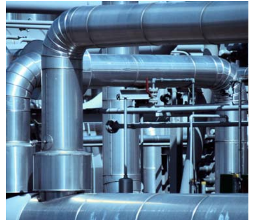
Ducting in a production facility.
